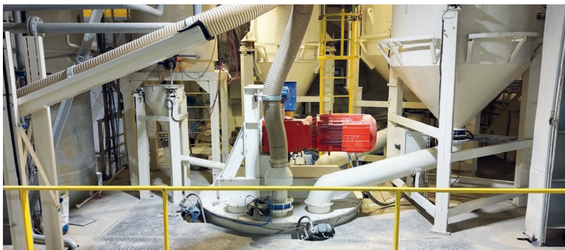
Overview of the Dual Pressure Cleaning System installed in an AAC mixer tower.
