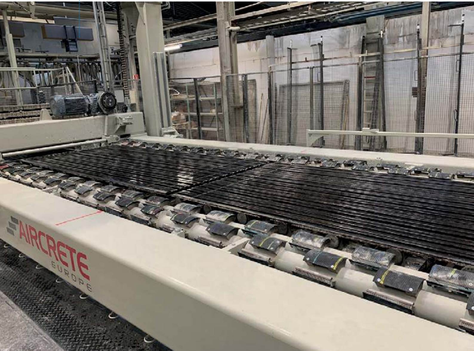
Fig. 4: The downtime for the project, including dismantling of the old equipment, installation of the new Aircrete Cross Cutter and commissioning was completed ahead of schedule.
