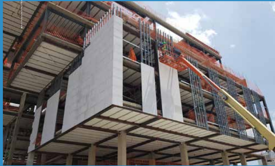
Fig. 1: A site application of reinforced products (floor and cladding panels on steel structure)
