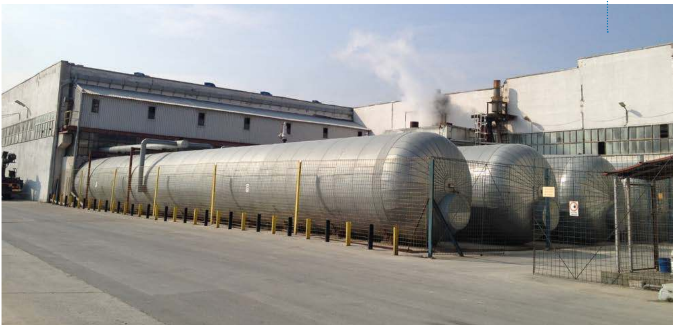
Fig. 1: Located in the city of Constanta near Black Sea, Celco has an annual production capacity of 400,000 m 3
