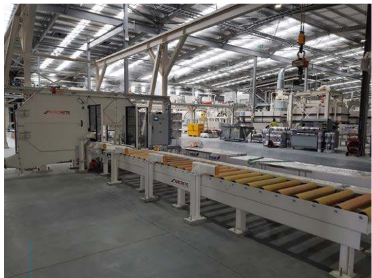
Fig. 4: Overview of the exit side of the system
