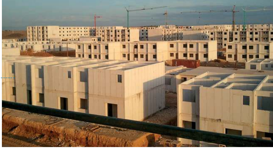
Fig. 2: The large housing projects in Sumbe, Angola are realized with AAC panels to create a modular, efficient and affordable building solution by Kora Angola [6].
