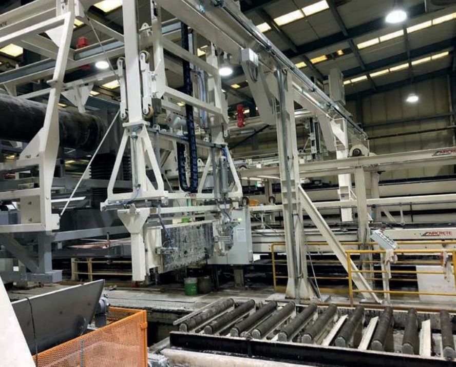
Fig. 2: The new fully automated end crust removal system.
