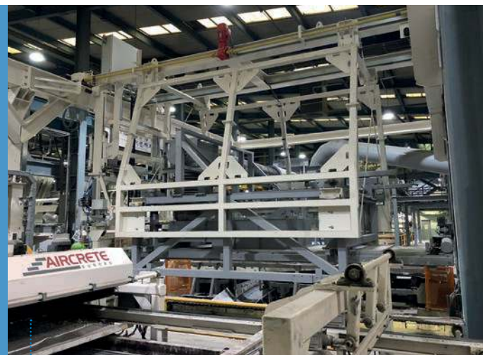
Fig. 3: The vacuum crane is repositioned and attached to a new vacuum hood crane for efficient top waste collection.
