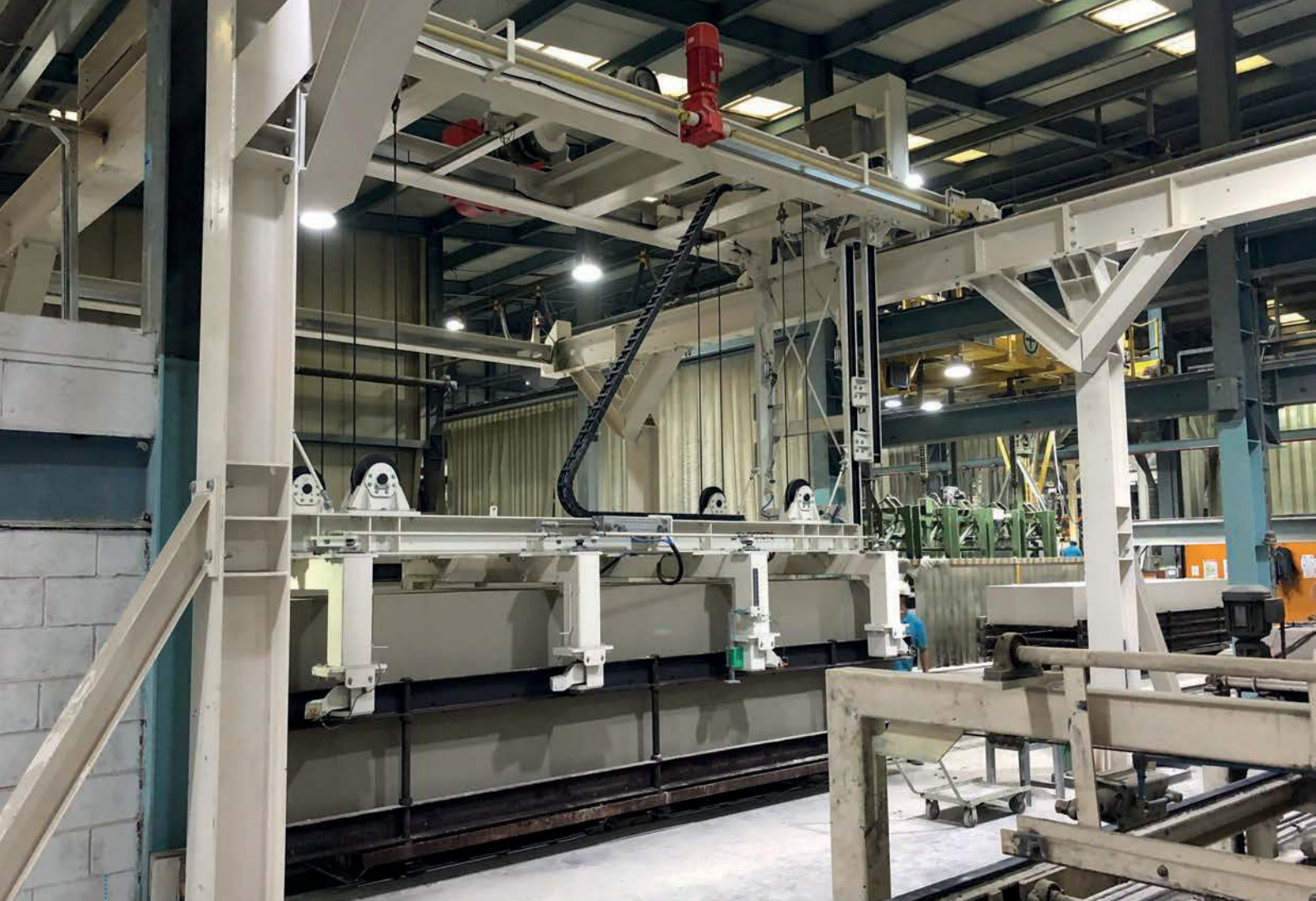
Fig. 4: The new frame stacking crane picks the cake automatically and stacks it two or three high as per the autoclave height.
