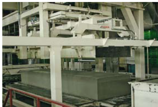
Fig. 6 The grabbing crane picks up the flat "green" cake for transport to the cutting machine.
