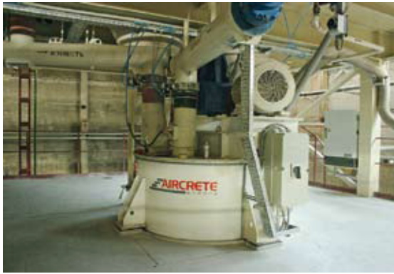
Fig. 3 Computer-based mixing control system for mixing and dosing of the raw materials.
