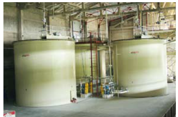
Fig. 2 This slurry is pumped into storage tanks and continuously stirred.
