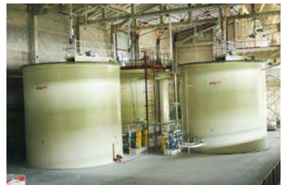
Fig. 2 This slurry is pumped into storage tanks and continuously stirred.
