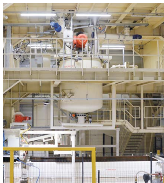
Fig. 5: Mixer and high-pressure cleaning nozzles visible flanged at its side.
